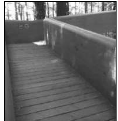
This walkway (pictured) at Lady Bird Johnson Grove will become ADA compliant
